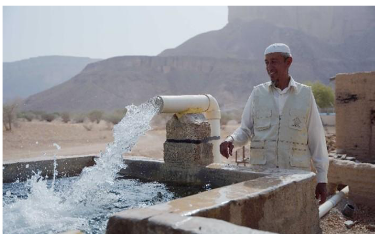
The solar-powered irrigation system for agricultural purposes project, Shibam district, Hadhramout | Photo Credit: UNDP
